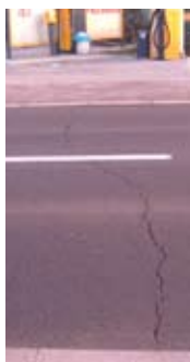
Fissure chaussée RN83 - Baume-les-Dames (Photo DDE)
